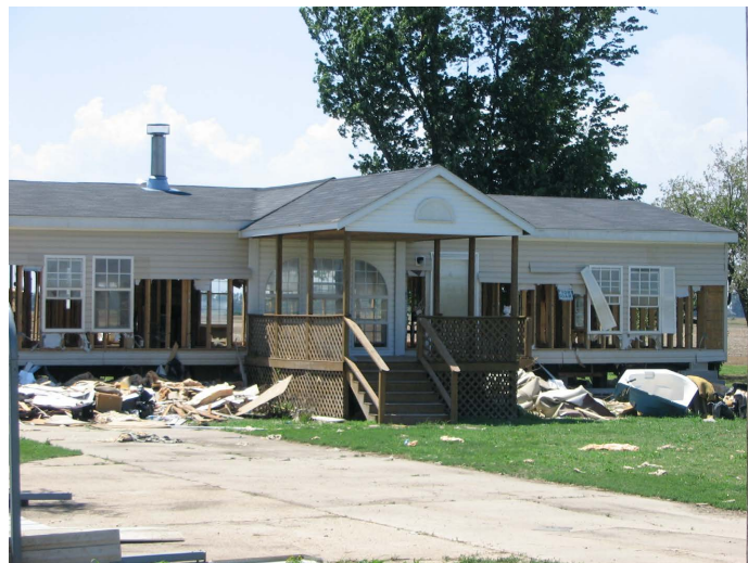
Figure 10. One of the 80 homes in the floodway was damaged by 2 to 3 m of floodwater in 2011.
