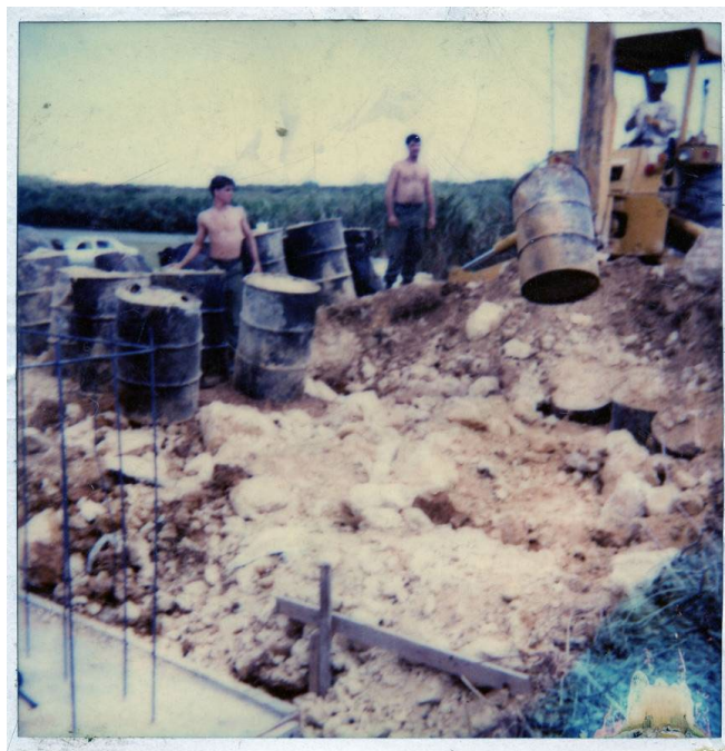
Figure 11. Repacking herbicide barrels and recovering buried barrels leaking into the ground. Reprinted with permission from editor of the Open Journal of Soil Science.
