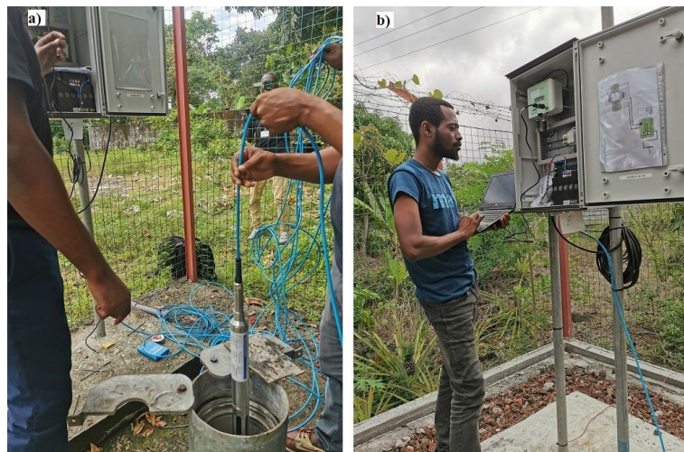
Photo 5. Device for measuring, recording and collecting piezometric data.
