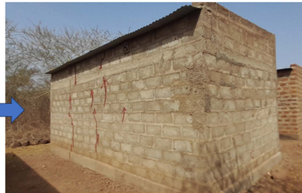
Photo 8: Exterior view of the breeze-block witness habitat in June 2023. Richard Z. June 2023
