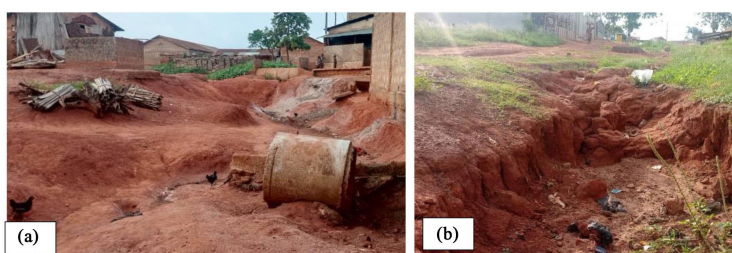
Plate 3. Condition of some damaged roads in the town of Pobè.
