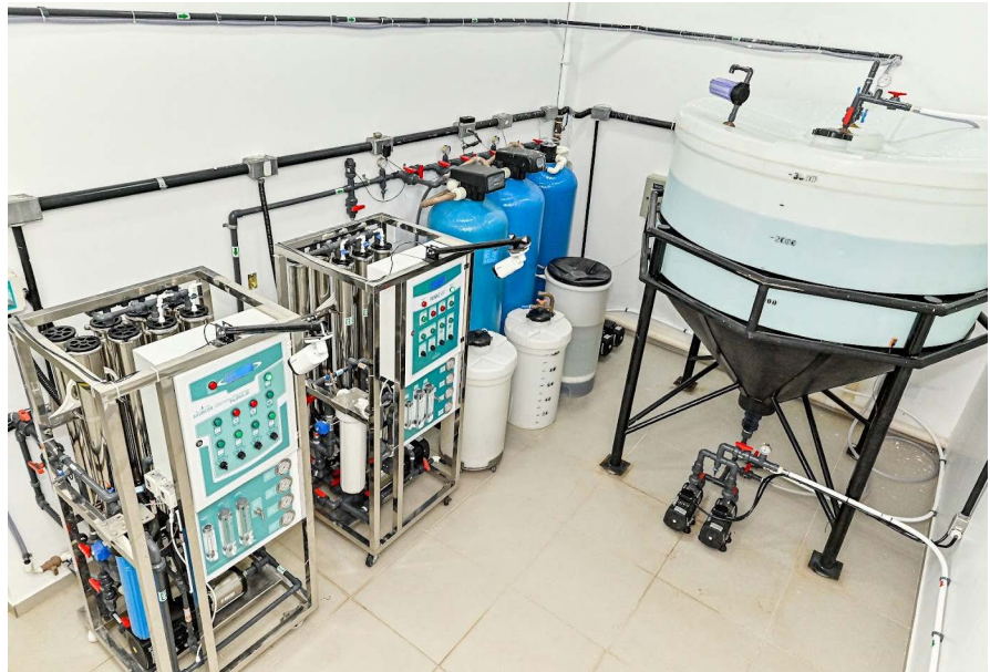
Figure 3. WTPic infrastructure, equipment arrangement and state of conservation of the nephrology clinic system, in 2024.
